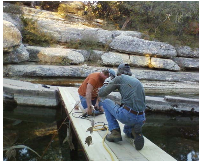
Garry Child and Darren work on the new bridge for the JW weir.
